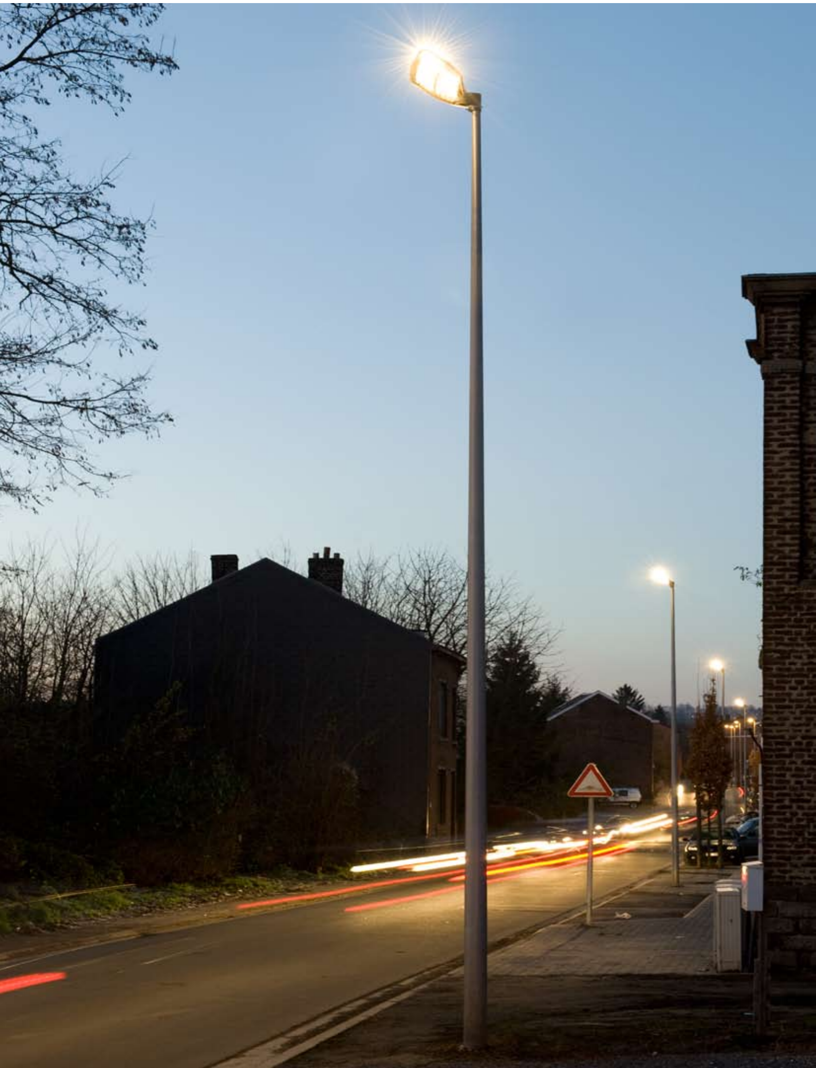
Belgium, Liège Vottem Five functional P186 have been installed in a tiny village. Welcomed by residents, who are unstinting in their praise, particularly for originality and the added security.
