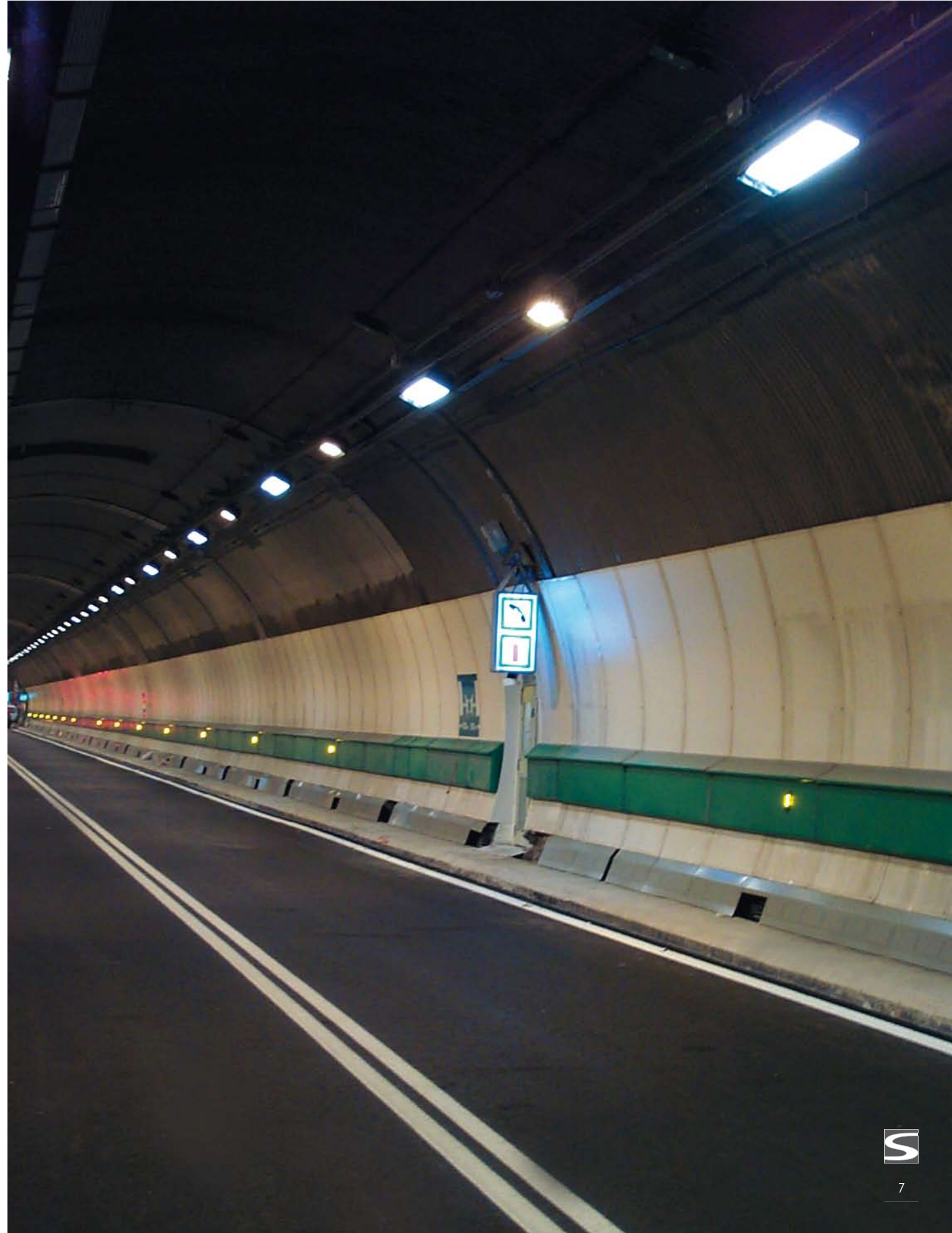
Italy, Aosta Mont-Blanc tunnel In tunnel application, LEDs serve mainly as guarantees of safety. 2654 LED guidance beacons were needed for the Mont-Blanc tunnel. In the near future, also for base lighting.
